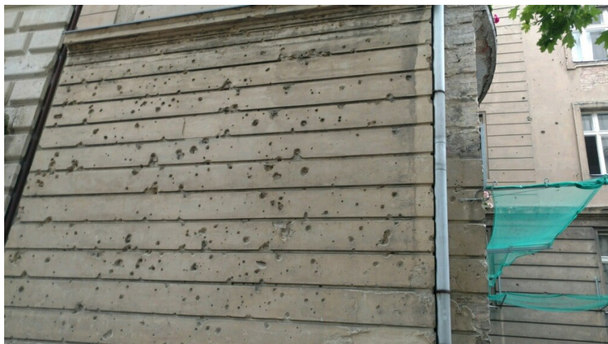
Bullet holes remaining in houses in East Berlin
